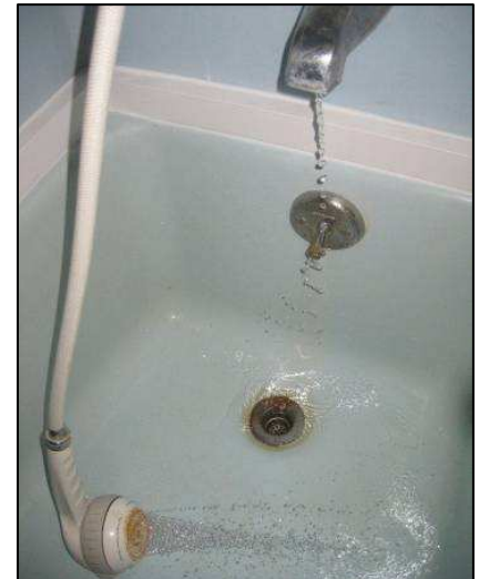
Figure 3: A leaking diverter allows water to flow out both the showerhead and the tub spout simultaneously.
